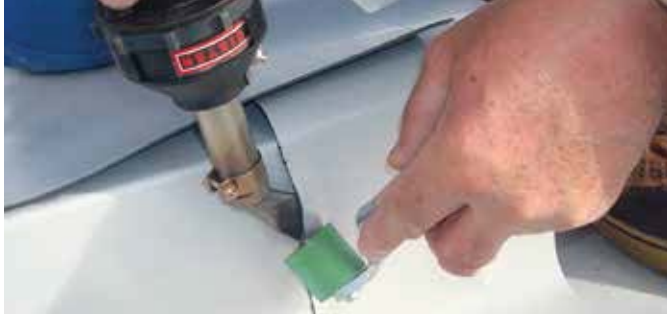
HOT JET S with angled nozzle welding a T-joint on the roof.
